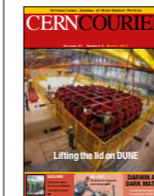
On the cover: The roof structure of protoDUNE being lowered into place at CERN in December. (Image credit: M Brice/CERN.)
